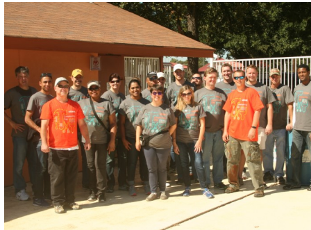
Vizient volunteers who were on the KIB team for "Community Day" spruced up the Lively Pointe Pool building with a fresh coat of paint.
